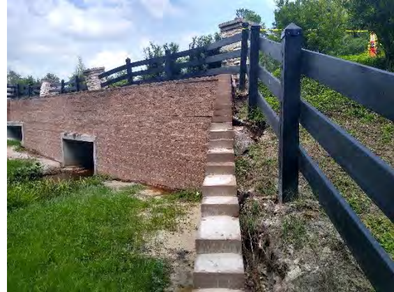
Image 3 – Erosion behind retaining wall
