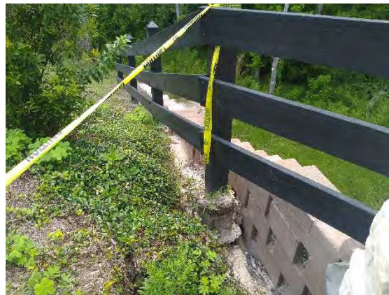
Image 4 – Erosion behind tapering retaining wall
