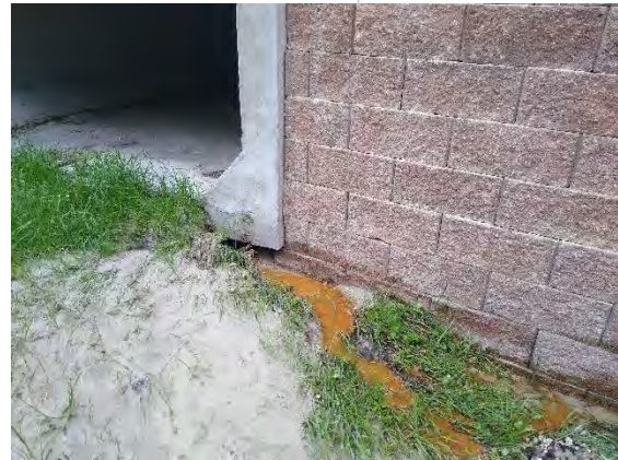
Image 6 – Erosion behind retaining wall
