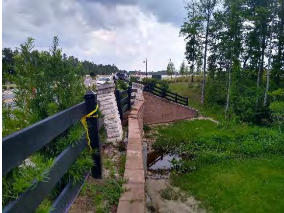
Image 2 – Retaining wall failure
