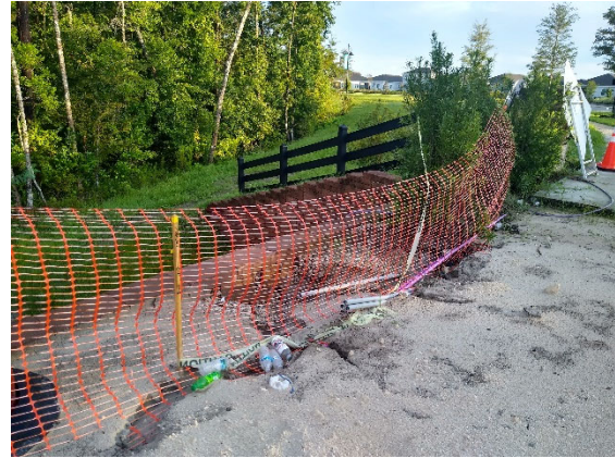
Image 10 – Erosion Behind Wall
