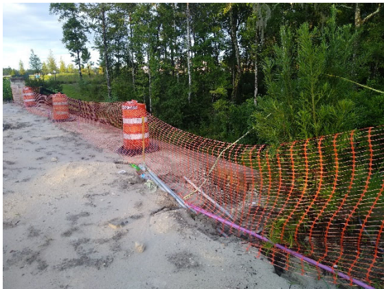
Image 11 – Erosion behind wall
