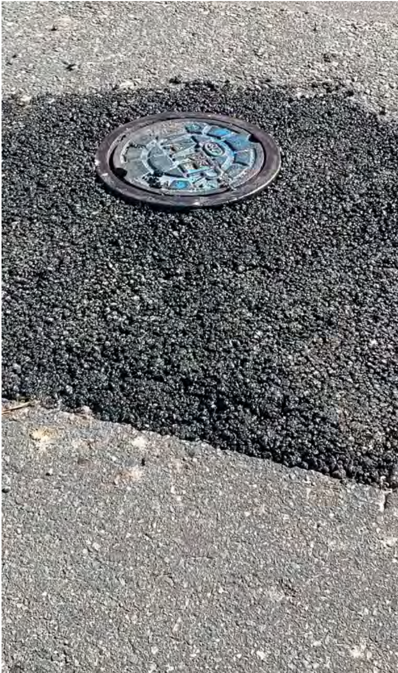
Patched Asphalt On Golf Cart Trail At Timberwolf Tr
