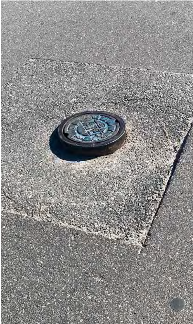
Patched Asphalt On Golf Cart Trail At Timberwolf Tr
