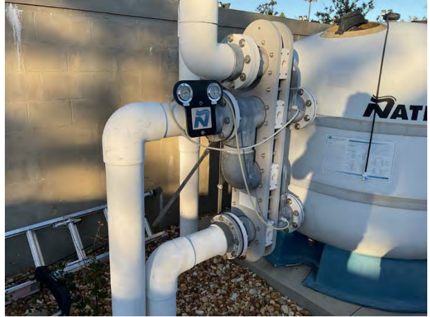
Pool mechanical equipment
