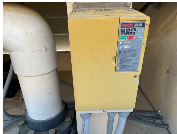
Pool mechanical equipment
