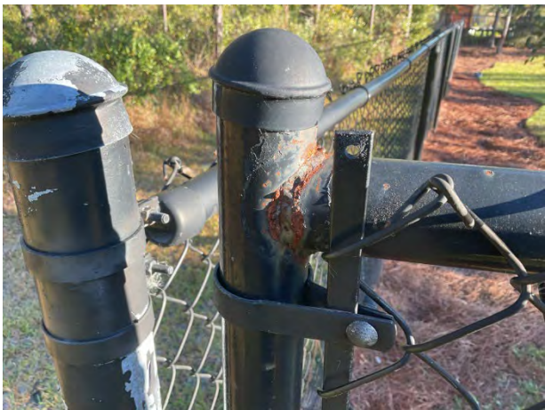
Fence post rust
