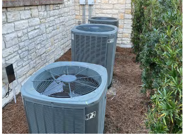
Split system condensing units
