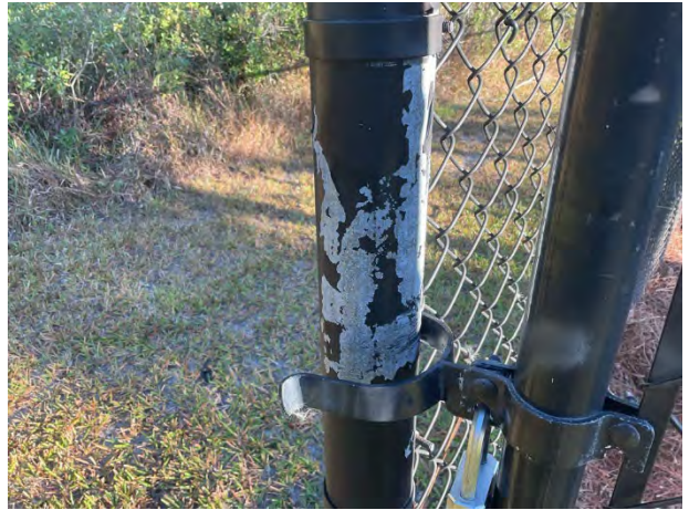
Fence finish deterioration
