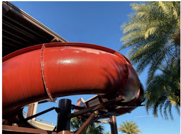
Water slide paint finish deterioration
