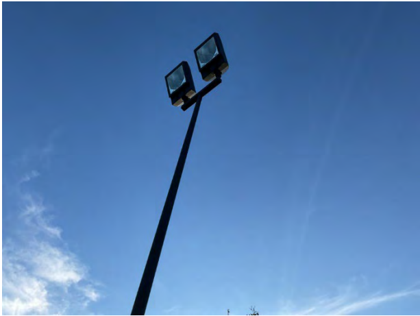
Light pole and fixtures
