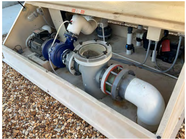
Pool mechanical equipment
