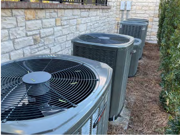
Split system condensing units
