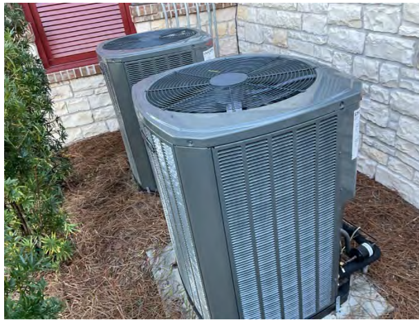
Split system condensing units
