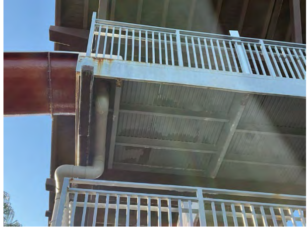
Rust at staircase and balcony
