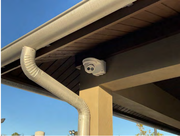
Security system camera
