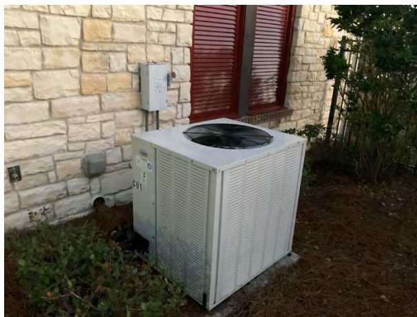
Split system condensing unit at entry pavilion
