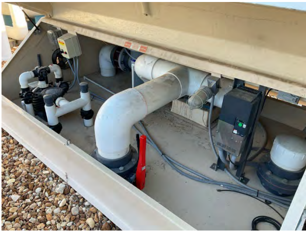
Pool mechanical equipment
