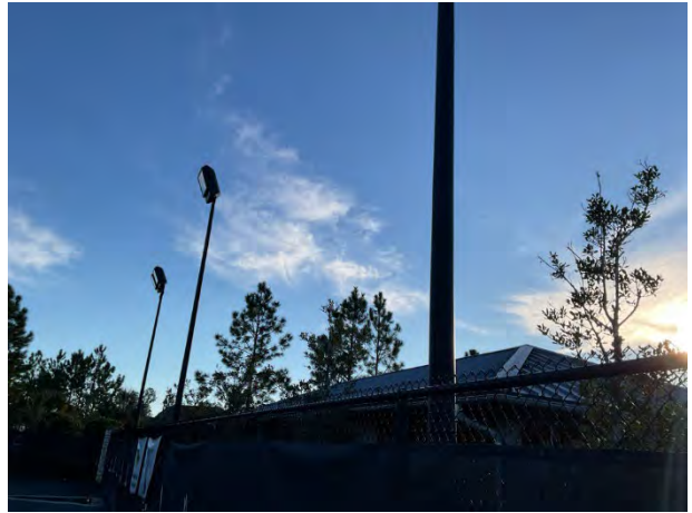
Light poles and fixtures
