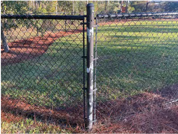
Fence finish deterioration
