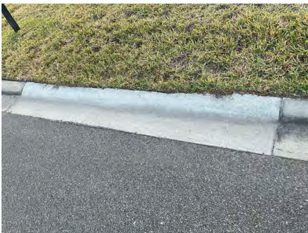
Concrete curb and gutter previous repair
