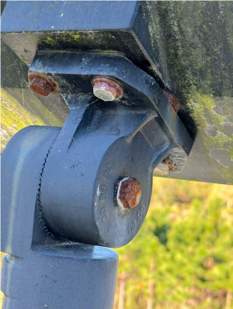
Tennis Court Light Fixtures Are Rusted Recommend Replacing Soon Created: Fri, 4/4/2025
