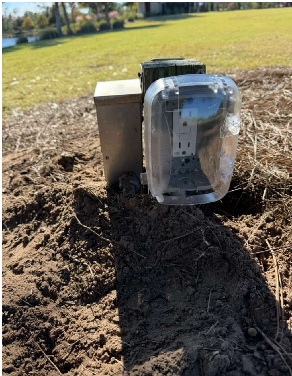
Installed GFI At Event Lawn
