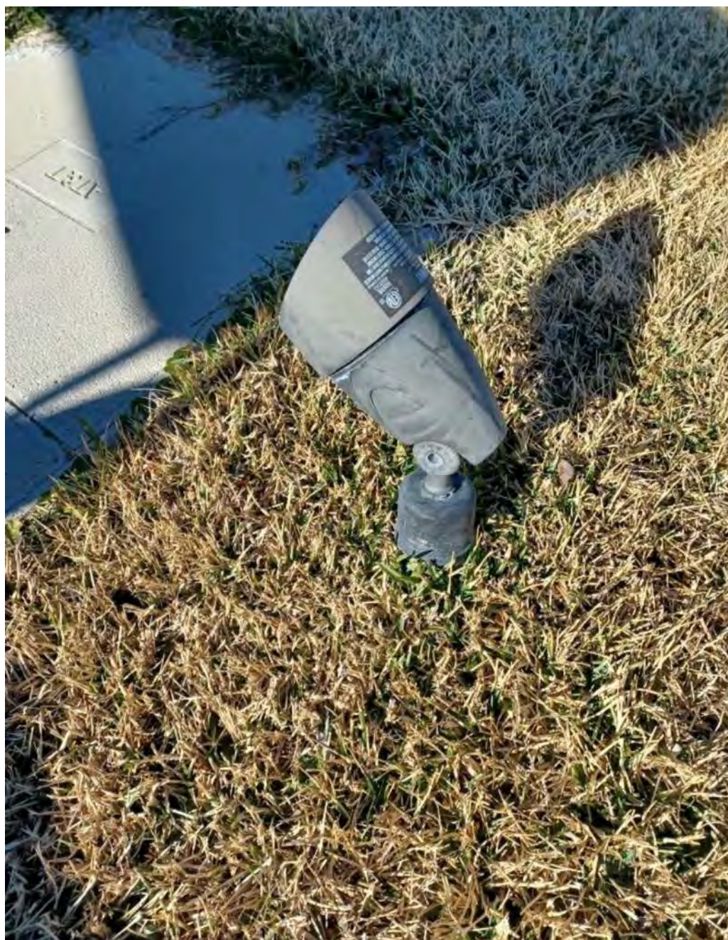
Replaced Light For Monument At The Hammocks Entry.
